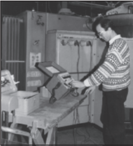
Oil-filled transformer being TTR tested upon receipt in plant. A full battery of tests would follow.
