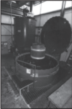
*Vacuum Pressure Impregnation* (up to 10 foot diameter)
