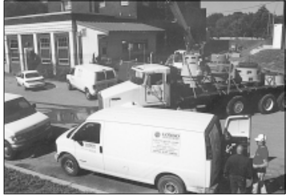
At the work site, LONGO crews were staged and ready to get our customer back in service. Note the number of our trucks at this one operation.
