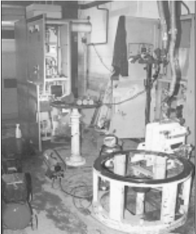
While one crew was working on motors, another was cleaning and repairing drives and switchgear. The major pumping station is being readied to go back on line.
