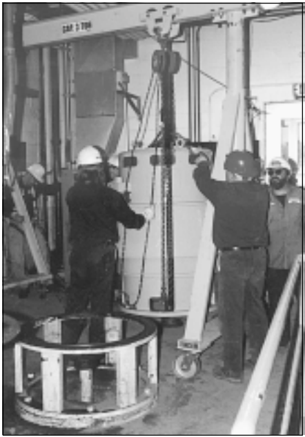
Working in confined quarters our crews used A-frame and hoist to maneuver large motor into position.
