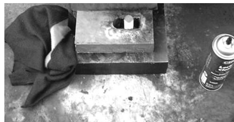
Preparing the mounting locations on site for the new foot print which included steel plates to ensure the proper alignment of the motor.
