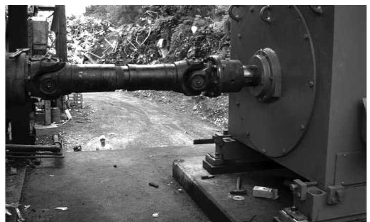
The shaft coupling had to be modified to match up with the shaft from the pulverizer.
