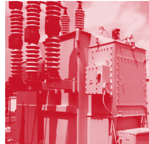
Top: Refurbished transformer
