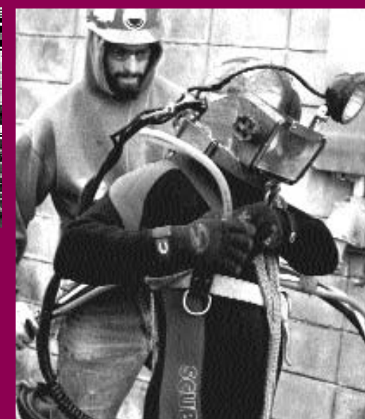
Divers were critical for the extraction, positioning and aligning the jack beneath the pump, adding the needed pressure to break the pump loose from the encrusted casing.
