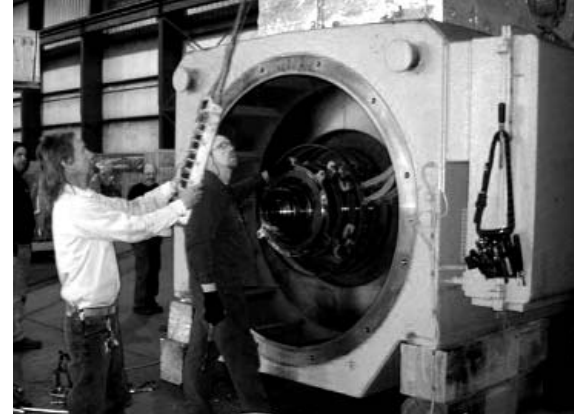
Left: Thanks again to the 100 ton crane, the removal of the rotor from this mammoth motor was done with the ease of doing a 500 hp motor back in the shop.
