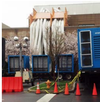
The rental ventilation equipment needed to substitute for the ruined fan and motor.
