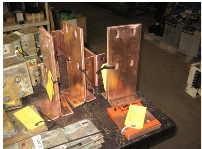
Just a few of the buss bar pieces as the corrosion from the salt water had to be aggressively removed.
