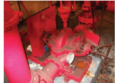
75 HP pump that needed overhaul and went to our Wharton Servicenter.
