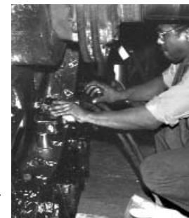
Mechanic and supervisor tighten rotor pole bolts using hydraulic calibrated torque wrench.
