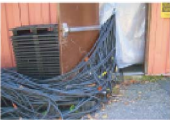
An extensive web of cables from the generator trailers had to be organized and channeled to the correct stations to re-energize the facility
