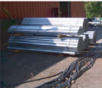
6,000 feet of conduit was needed for the cables to replace main buss running through the building. Obtaining a replacement buss would not have been time effective.
