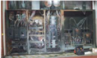
The extent and heat of the fire is evident from the damage in the switchgear units. However, note the plastic mirrors above the cabinets. Electrical fires can be very unusual in how they do their damage.
