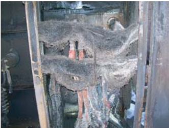
Remnants of the transformer that ruptured and sent burning oil into the switchgear area.
