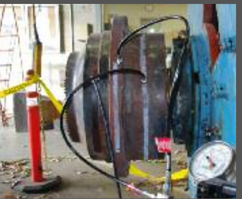
Once we were setup and pressurized we waited and we waited...nothing. The initial pressure, 15,000 psi, was a little low. When we corrected that up to the prescribed 45,000 psi it worked just fine! be aware of, otherwise the bearing itself can be damaged. A differential of 85 degrees C between the bearing and the shaft is usually sufficient to remove or mount a bearing. When the differential approaches or exceeds 125C the bearing itself can be damaged.
