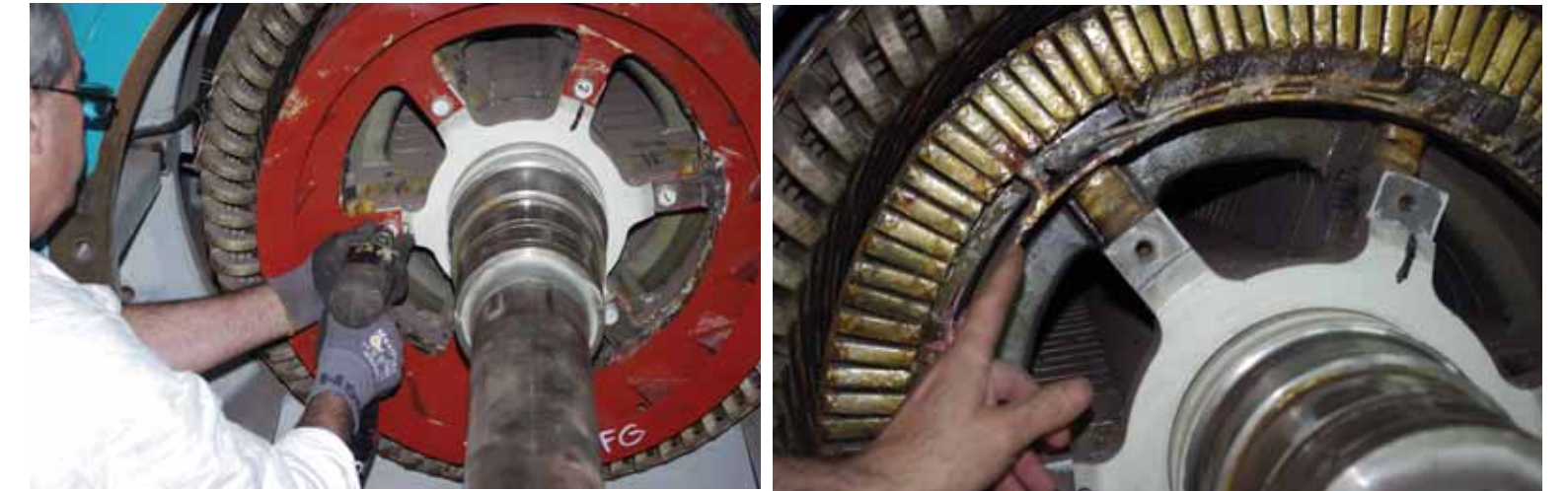
The procedure begins with the dismantling of the hub. Once the area is open, and available, the Wye ring can be examined by eye to find any faults. A specific infrared procedure is available to ensure "invisible" breaks are also caught and repaired.
