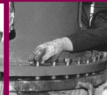
With each part cleaned, repaired, or replaced the reassembly was relatively trouble free. There is always the concern that even these massive elements could go out of round or distort after years of confinement, but that was not the case. Outstanding crane work and a delicate touch had parts easing into place on the first try.
