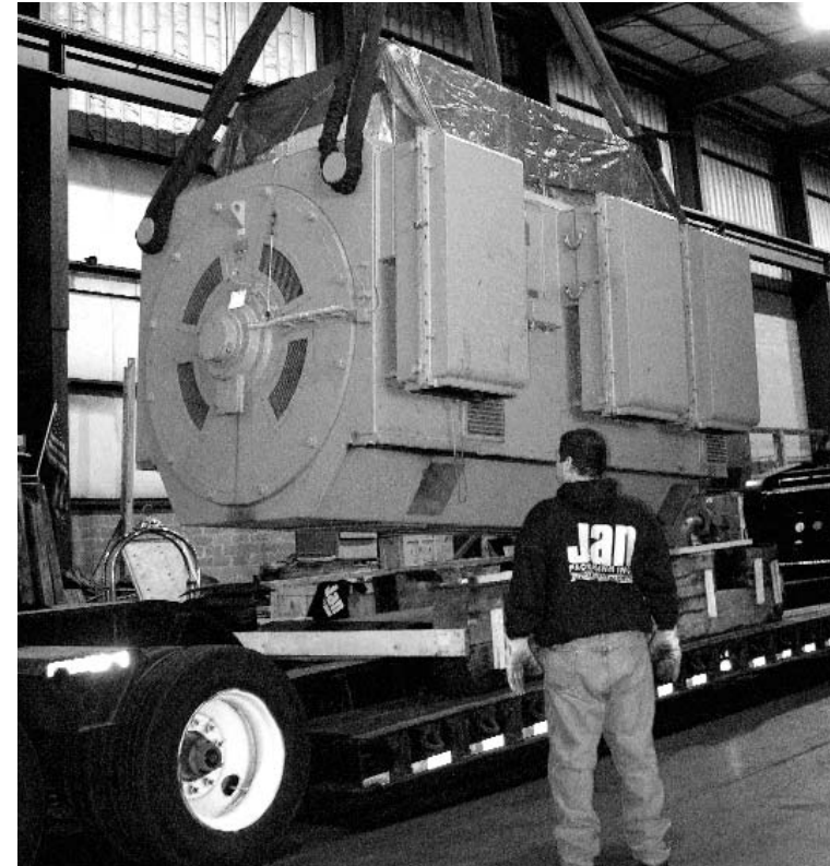
Below: The rigging company, with its 100 ton crane, made the unloading and positioning of the motor a very secure operation. While the motor was huge, one of the crew stated, "I thought it would've been taller". The replacement exhaust fan unit was taller than the older one shown here. As such it had to be shipped separate of the motor to insure that it did not hit any of the overpasses, etc.
